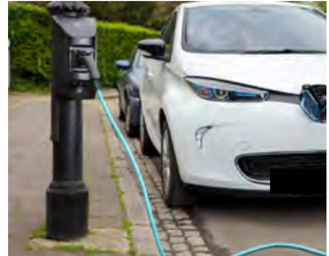
Figure 80: Example of on-street electric vehicle charging points.
