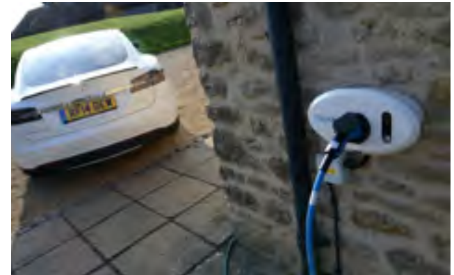
Figure 82: Example of off-street electric vehicle charging points.
